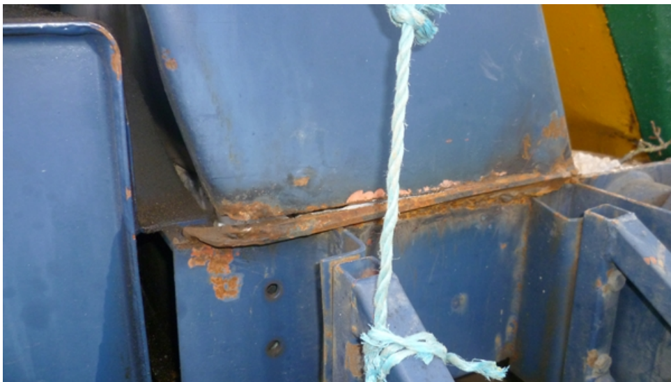
Figure 11 – Crack in lifting equipment
