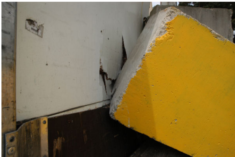
Figure 14 – Damage to headboard (Image supplied by TRL Ltd)
