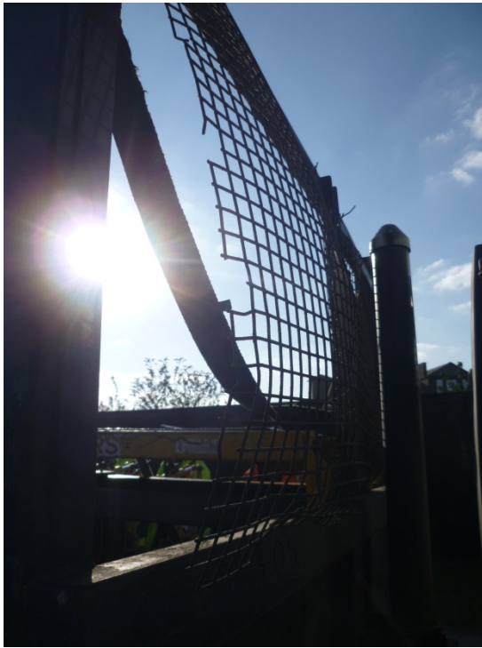
Figure 8 – Damage to wire mesh headboard
